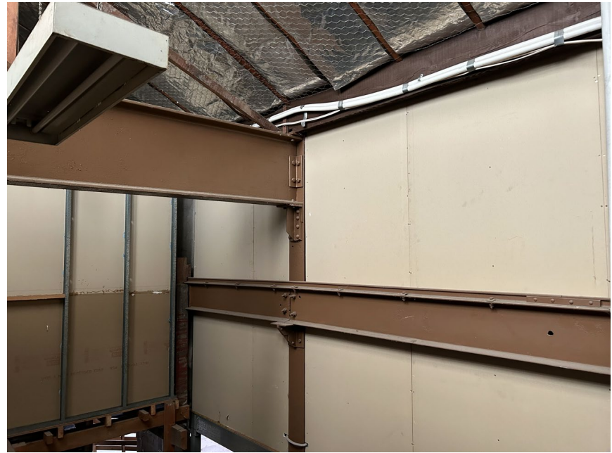
existing structural columns and beams to be retained, with steel hoist beam (centre) to be removed
